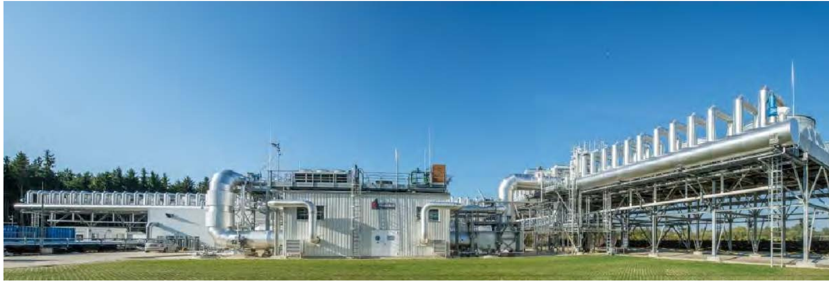
Turboden, 5.6 MWe geothermal ORC Turboden plant for Hochtief Energy Management Kirchstockach – Munich, Germany
